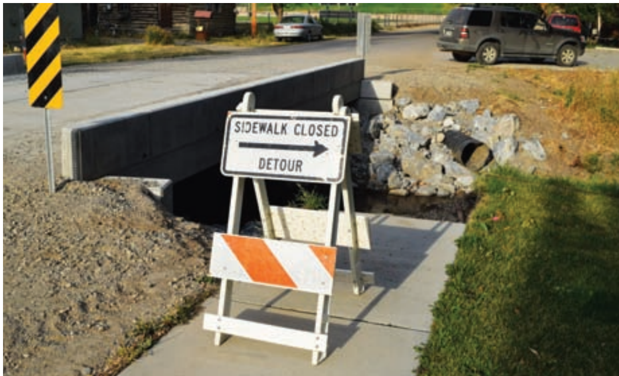
ABIGAIL DENNIS/THE MADISONIAN The Moore Creek culverts and bridges still require finishing work.
