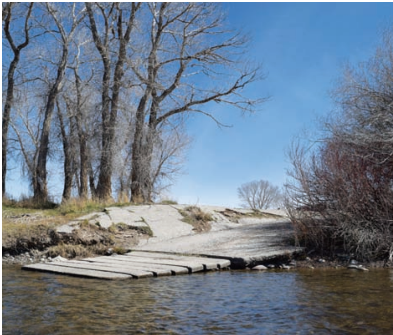
ABIGAIL DENNIS/THE MADISONIAN The boat ramp at Varney Bridge fishing access site needs to be replaced because it is "crumbling" and a "hazard," according to FWP's Cheryl Morris.
