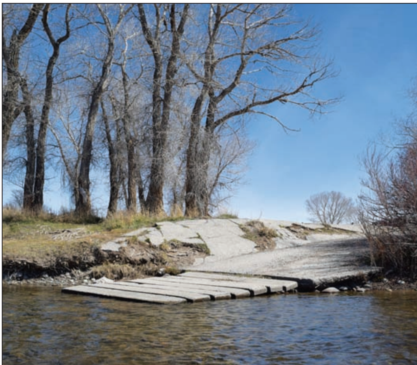
ABIGAIL DENNIS/THE MADISONIAN Construction to replace the Varney Bridge fishing access site boat ramp is slated for later this spring.
