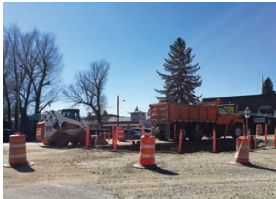
ABIGAIL DENNIS/THE MADISONIAN Construction on the first culvert is being done in three phases, right now, the contractors are working on the culvert as it passes under Main Street.
