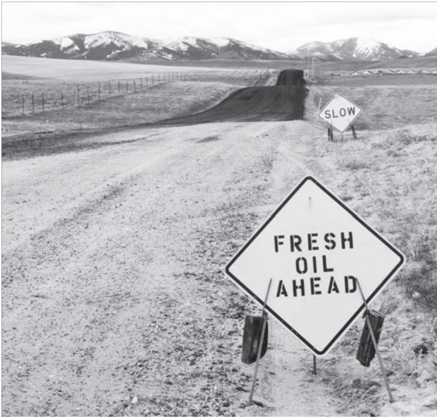
Harrison Lake Road received a makeover this last week. Two and a half miles of road were resurfaced. The road resurfacing project is a part of county-wide effort to improve various roadways in Madison and Ruby Valley. The road crews of Madison Valley have also teamed up with Jefferson County on some projects since some roads overlap county lines.
