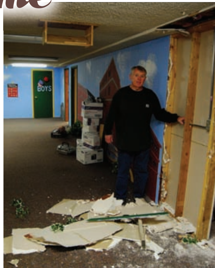
Charles Tucker standing at the first area of demolition in the basement, the future Youth Center.
