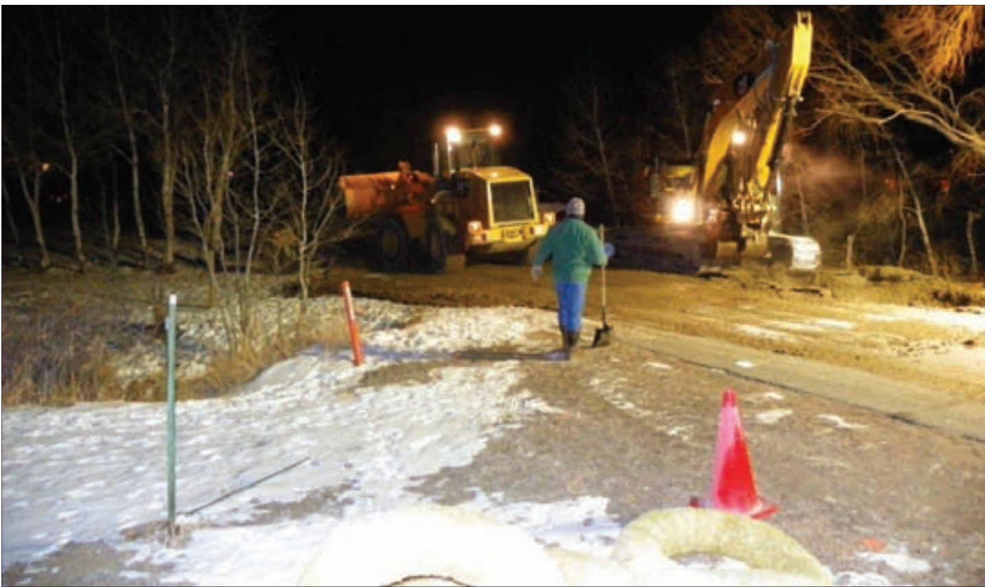
Crews worked late into the night to mend a broken water main on Armitage Street by Moores Creek.
